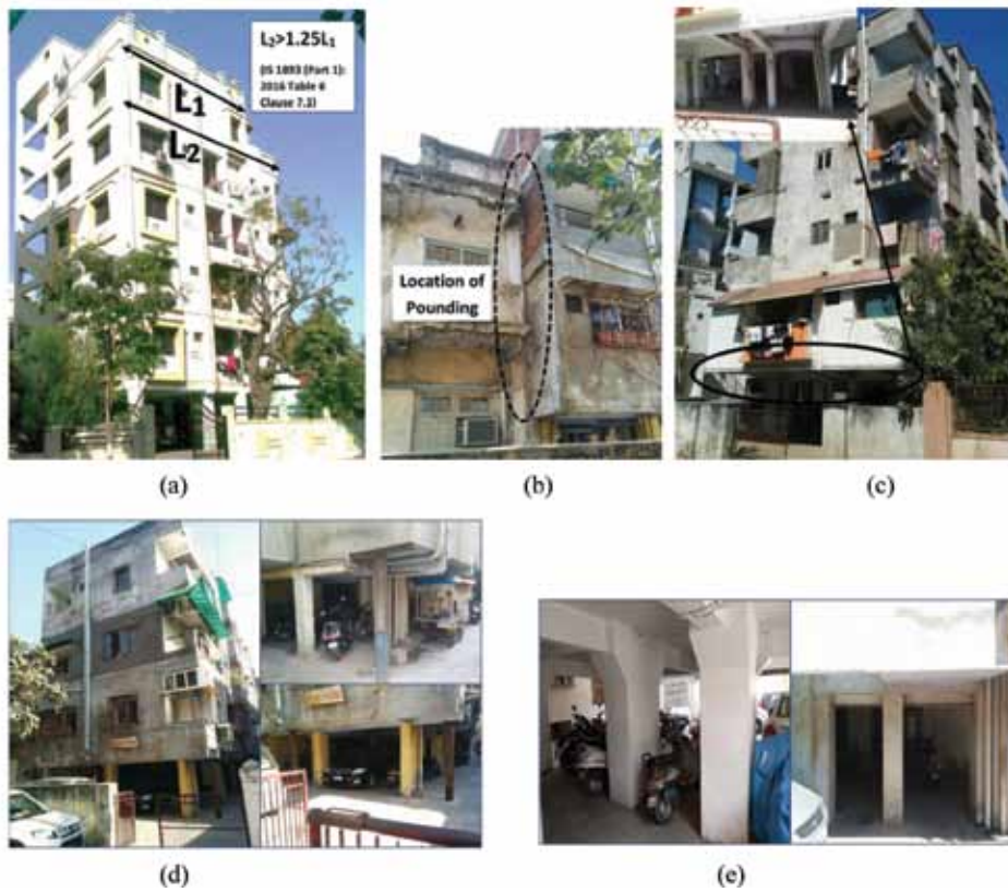
Figure 6. ((a) Vertical setback, (b) Possible location of occurrence of Pounding, (c) Overhang in form of jutting out balconies, (d) Poor quality of construction (e) Retrofitting through Column jacketing and steel I beam).
