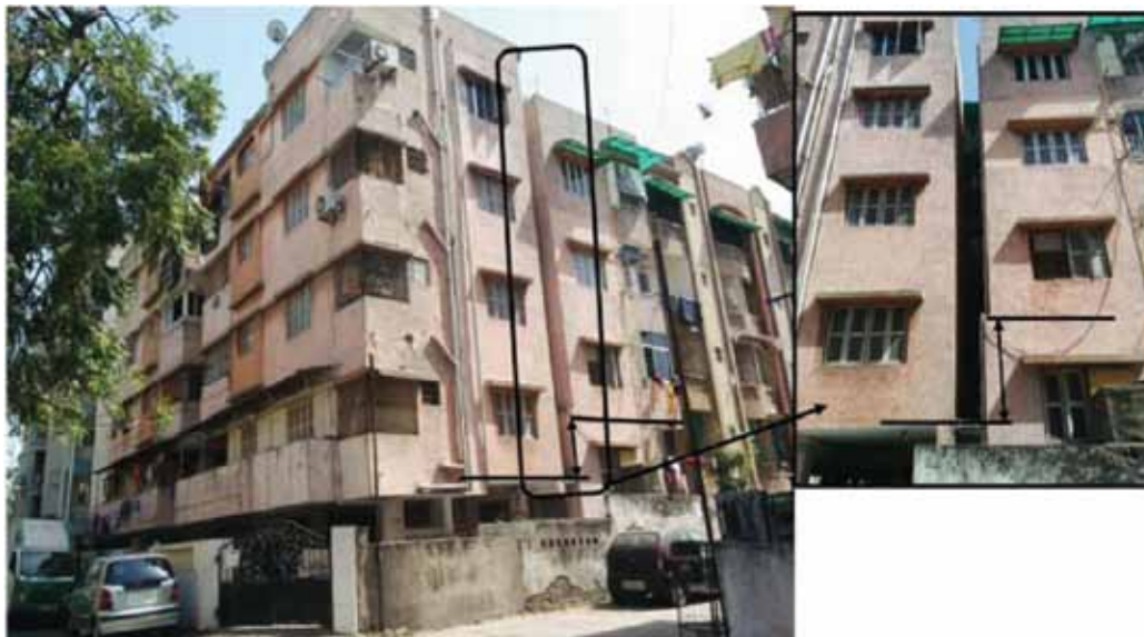
Figure 5. Partial soft storey
